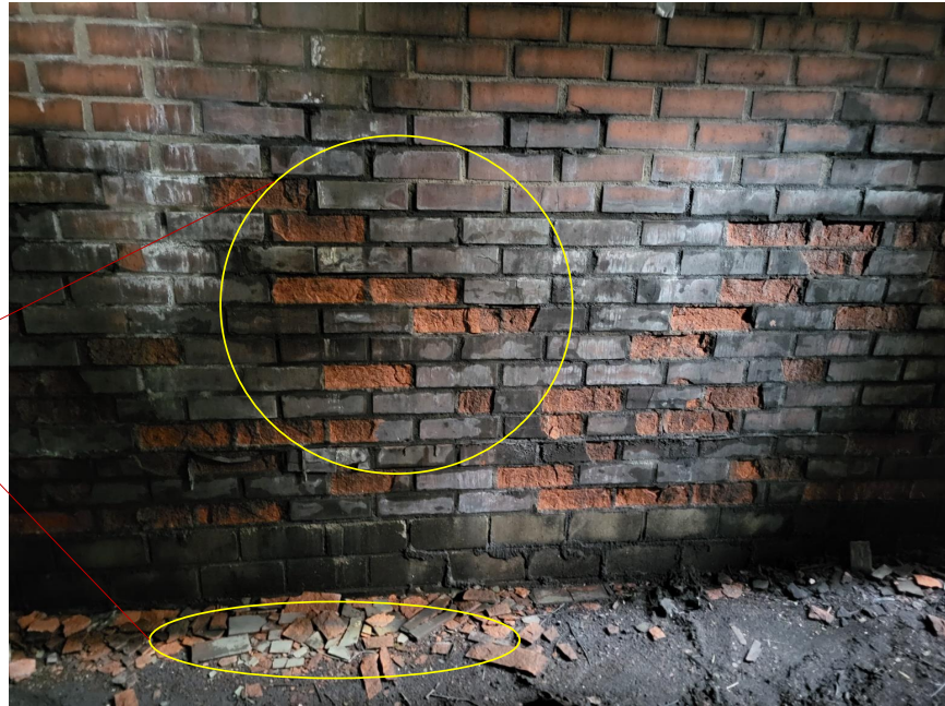
Fig 8: Bricks spall off due to water absorption on north side of towing vehicles IV and V , photo captured by Sooraj Nair, 2024.
